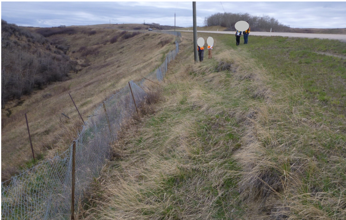
Photo 4 Slide 3 – Back scarp measured to be 4.2 m from asphalt (no change from 2018). Fence displacement down slope. Pole in slide area leaning approximately 5° downslope. Photo taken facing west on May 10, 2019.
