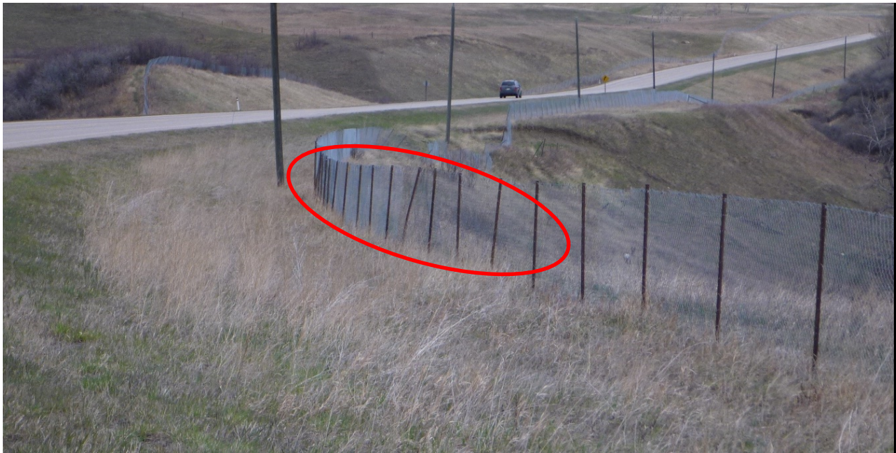
Photo 3 Slide 2 – Fence displacement at the head scarp (red circle). Pole in slide area leaning approximately 5.6° downslope. Photo was taken facing north on May 10, 2019.
