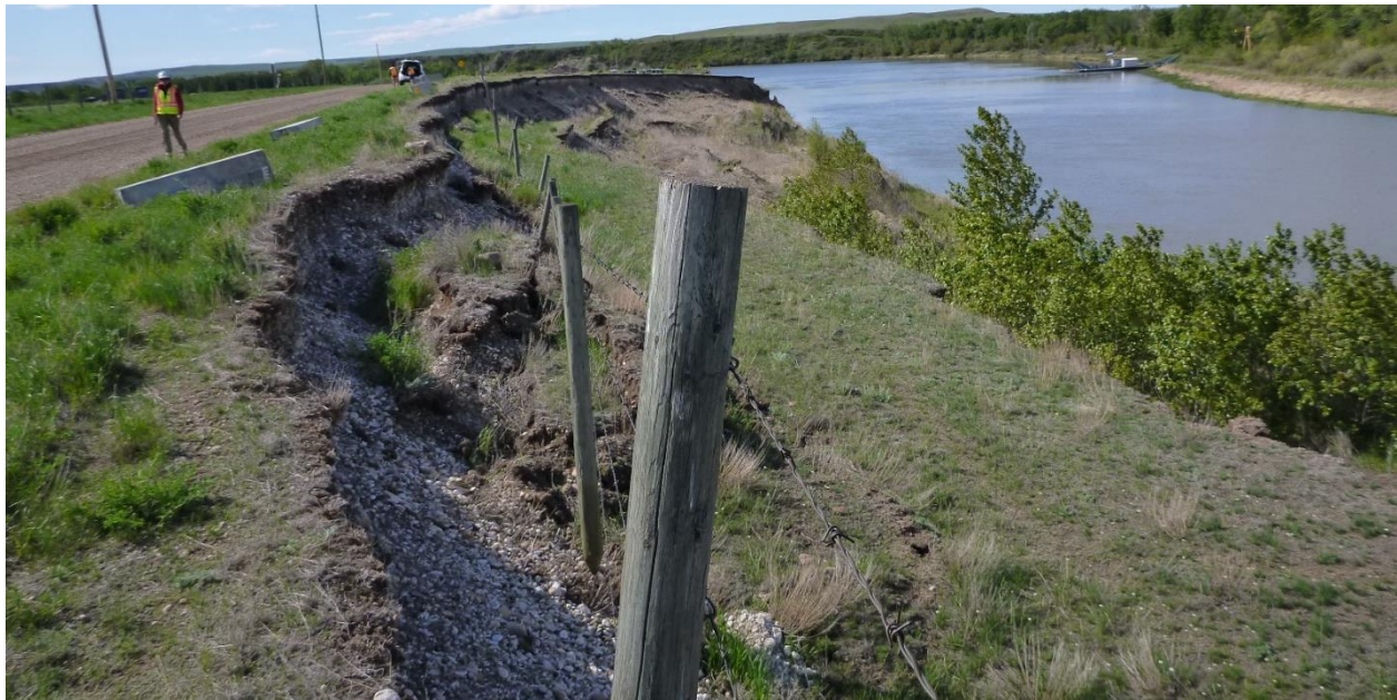
Photo 5 Concrete barriers have been placed along the length of the slide between the head scarp and the highway. Photo taken May 29, 2024, facing southwest.
