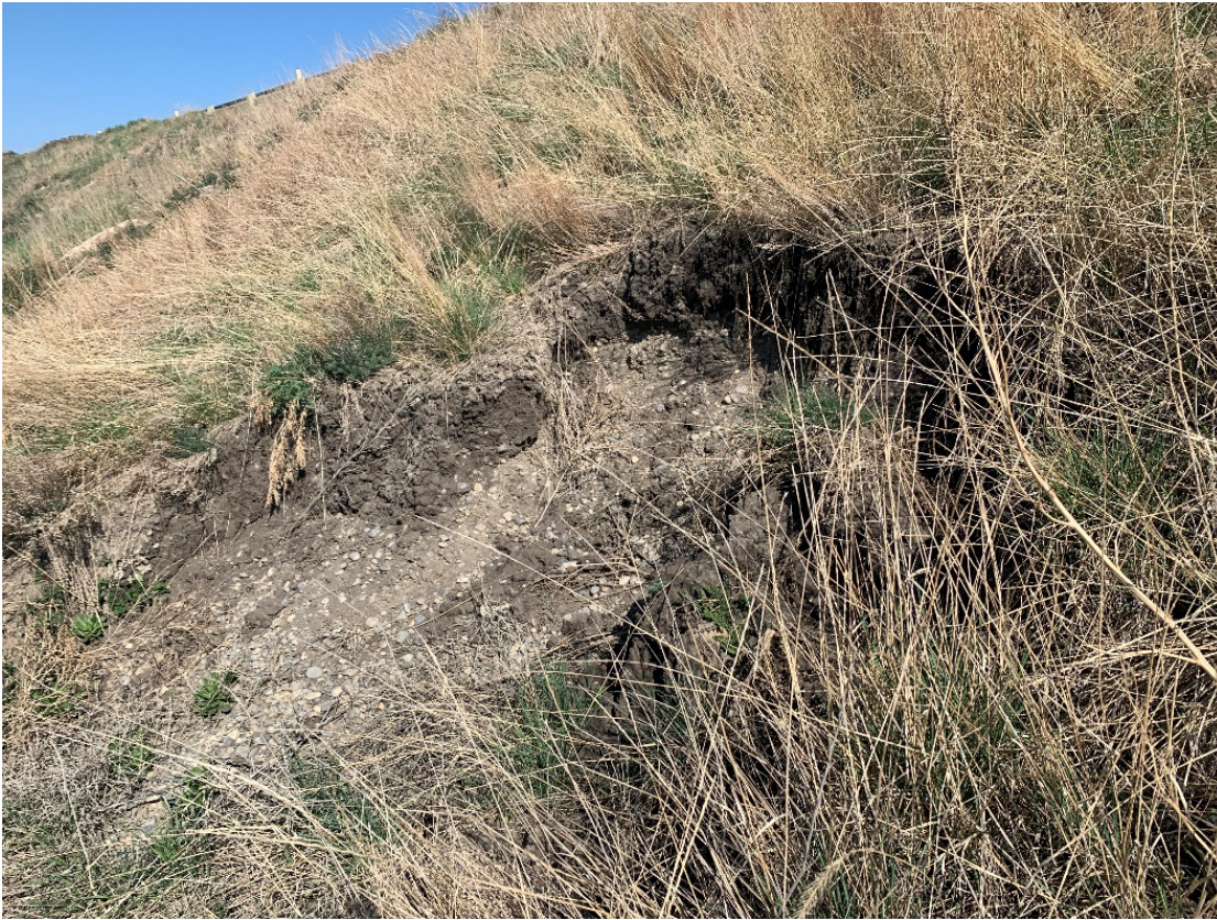
Photo 6 South side of highway – Visible granular fill and displaced vegetation near fence line of the repaired section. Photo taken facing west on May 12, 2023.
