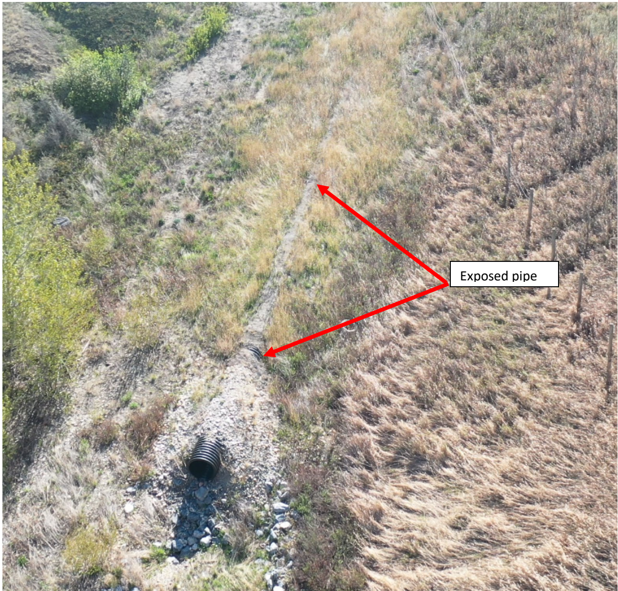
Photo 3 North side of highway – slope drain. Note exposed pipe at two locations. Photo taken facing east on May 12, 2023.
