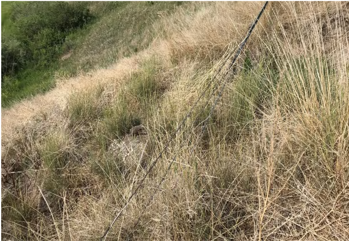
Photo 5 South side of highway – Displaced mid slope fence line due to failure of 2018 granular embankment repair. Photo was taken facing west on July 7, 2021.
