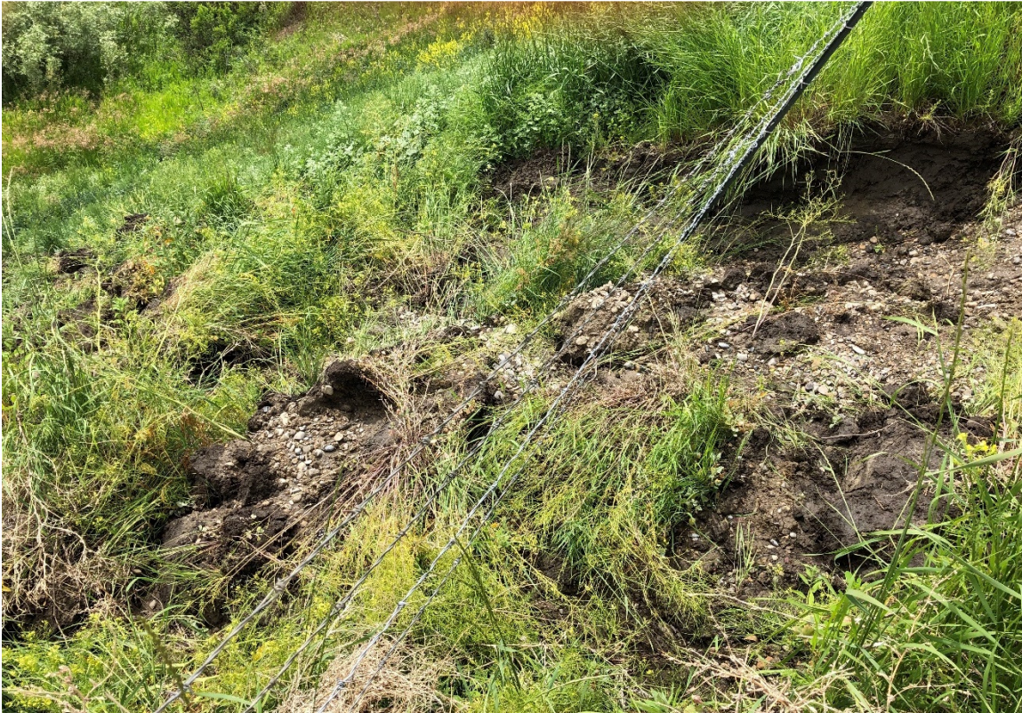
Photo 7 South side of highway – Failure of 2018 granular embankment repair adjacent to the fence line. Photo was taken facing west on July 8, 2020.
