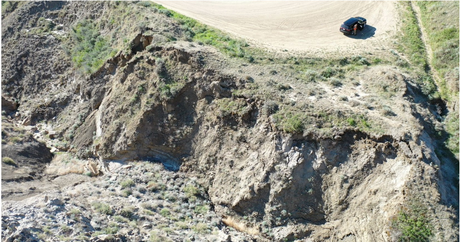
Photo 2 Aerial photo of the north side of the highway at the S040 Dorothy Sinkholes site. There is ongoing erosion of the north slope and the erosion has exposed bedrock at the toe of the slope/ditch bottom. Photo taken May 31, 2022, facing southeast.
