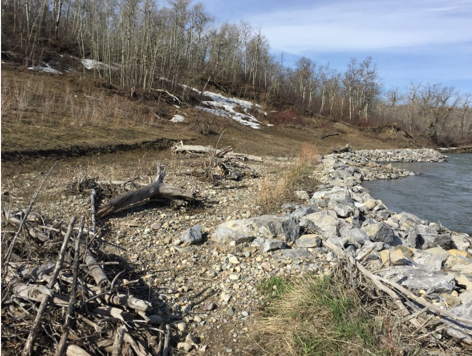
Photo 5 High water since the previous inspection in 2017 has deposited tree debris and caused some erosion at the toe of the slope. Photo was taken facing southwest on May 3, 2018.
