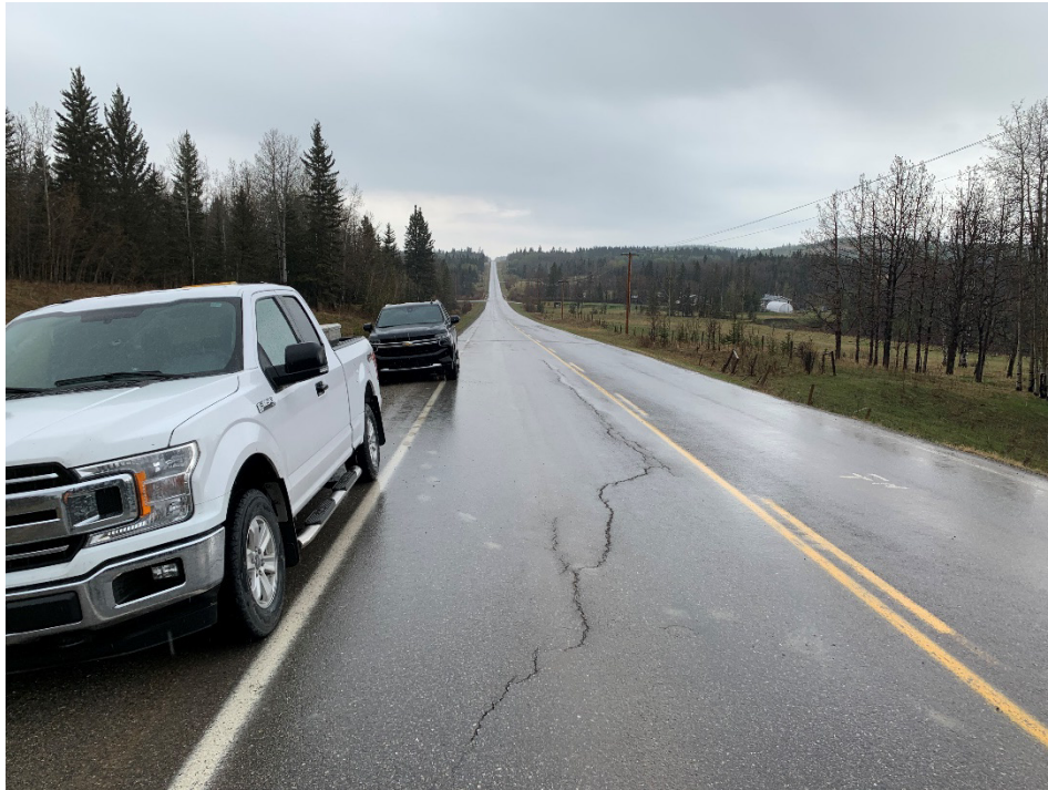
Photo 3 Pavement cracking extends to centreline. Photo was taken facing north on May 9, 2023.
