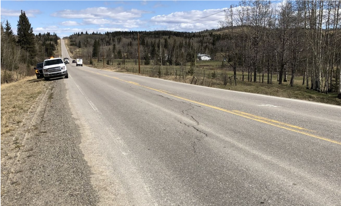
Photo 5 Longitudinal pavement cracking in the west (southbound) lane. Photo taken May 16, 2022, facing north.
