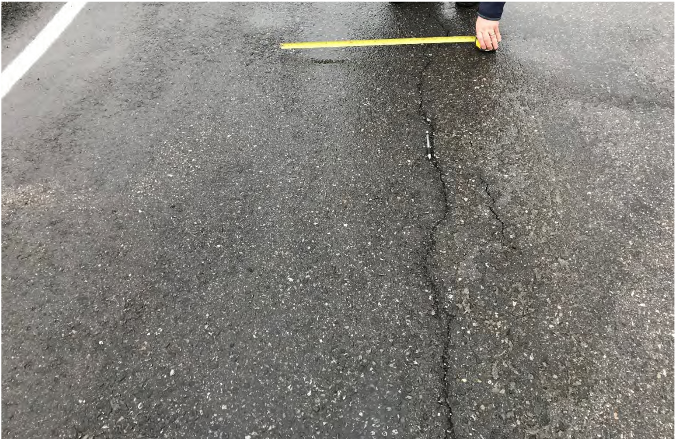
Photo 3 S031 Site II – Pavement cracking halfway into the southbound lane. Photo was taken on July 5, 2021.
