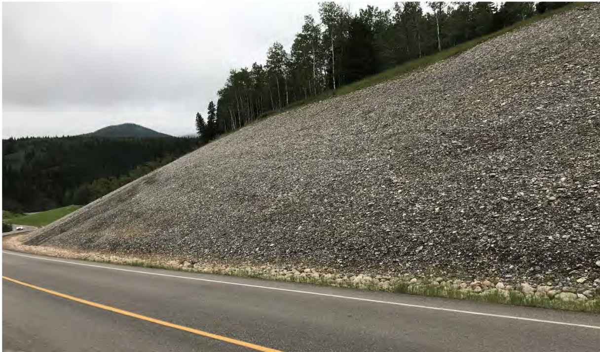
Photo 3 Unvegetated cut slope from highway realignment. Photo was taken facing west on July 5, 2021.
