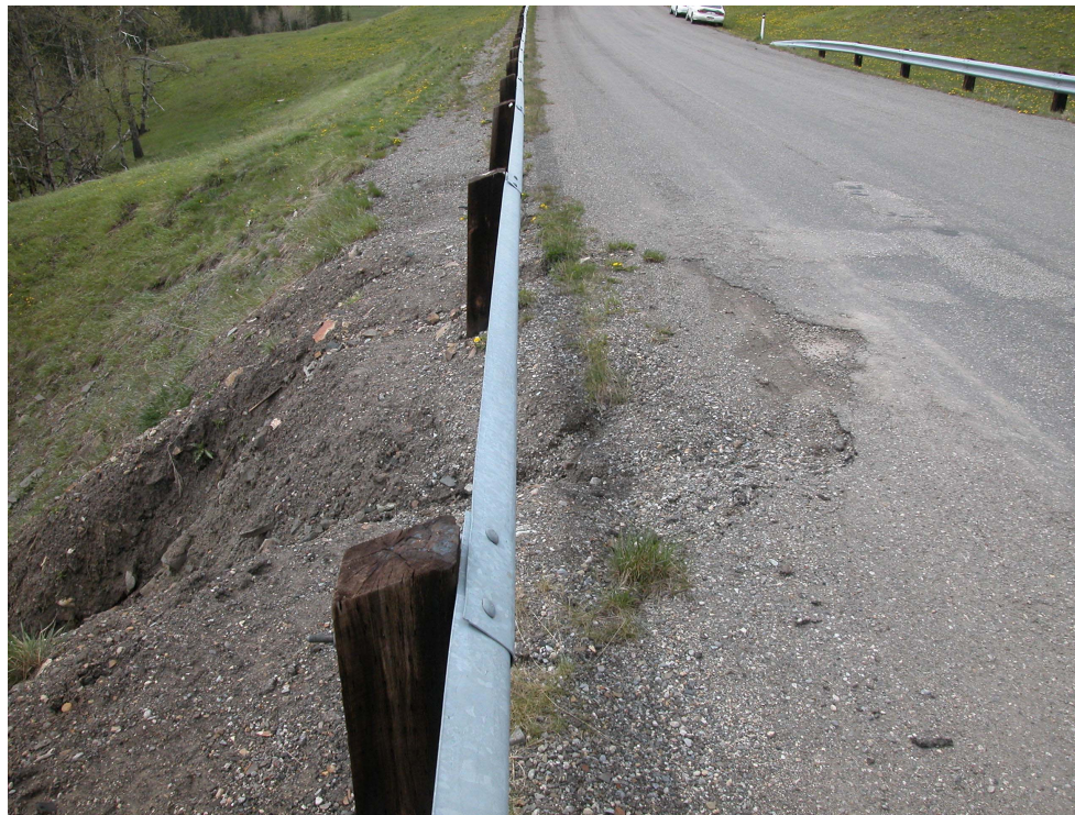
Photo S13-1 (upper left) – May 2004 – gully erosion retrogressing into the south edge of the road surface. There has been a slight retrogression (estimated less than 5 cm) of the erosion further back into the road since the July 2003 inspection. Compare with Photo S13-2.
