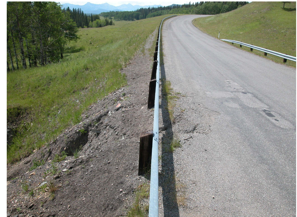
Photo S13-2 (upper right) – July 2003 – same area as shown in Photo S13-1, as seen during the July 2003 inspection.
