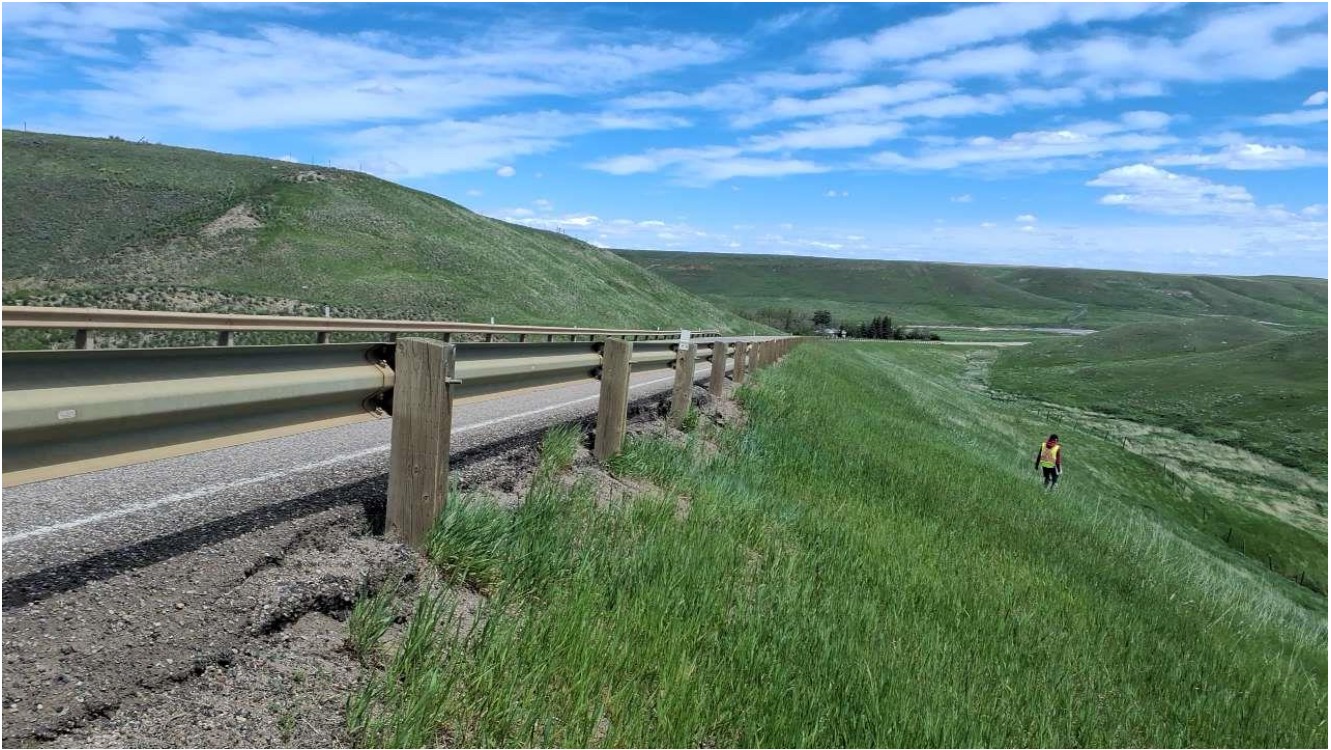
Photo 6 Head scarp at the edge of the pavement. Loss of pavement support over approximately 20 m length. Photo taken facing west on May 29, 2024.
