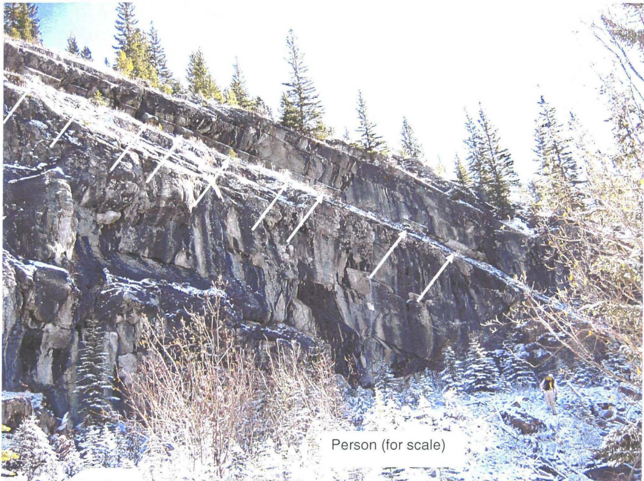
Photo 4 (bottom) – Concrete buttress blocks installed along a bedding dip slope above Highway 40. (Locations of blocks marked with white arrows.) Note the person in the lower right hand corner of the photo for scale. Please also see Figure D2 for an illustration of how the buttress blocks were constructed.
