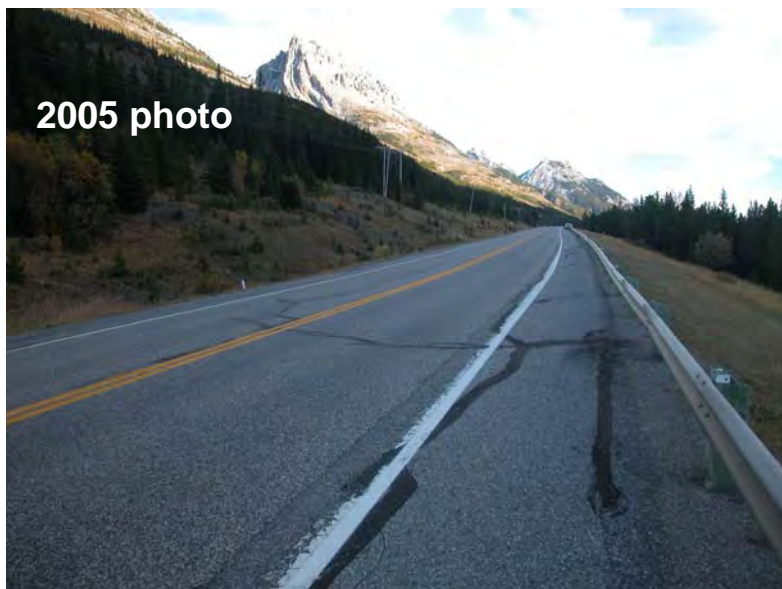
Photo 4 (bottom) – 2005 Fortress Junction Road Cracking Site The same area as shown in Photo 3, as it appeared during the 2005 inspection.
