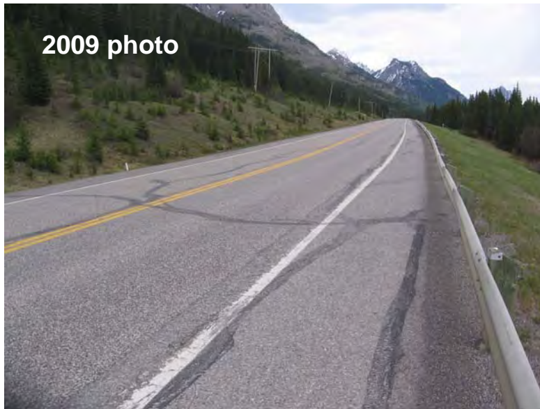
Photo 3 (top) – June 2009 Fortress Junction Road Cracking Site Facing southbound across the settlement and cracking area in the southbound lane. The pattern of the cracking and downdrop is suggestive of slumping of a segment of the downslope lane, however when compared to Photo 4 from the 2005 inspection it does not appear that the damage to the road surface has worsened in recent years.
