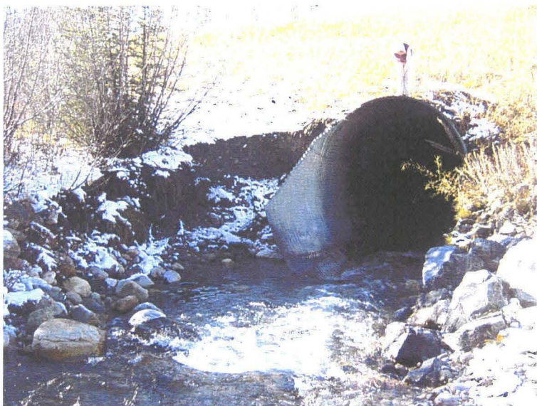
Photo 1 (top) – October 2005 – Culvert inlet at the toe of the east highway embankment sideslope at the Lusk Creek crossing. Peak flows earlier in 2005 have caused soil erosion at the toe of the sideslope immediately south of the culvert inlet (on the left side of this photo).
