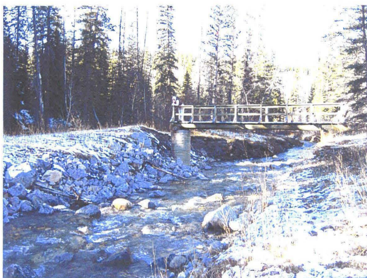
Photo 2 (bottom) – Footbridge across Lusk Creek, approximately 50 m downstream of the culvert at Highway 40. The south end of this bridge was washed out during peak flows in June 2005.
