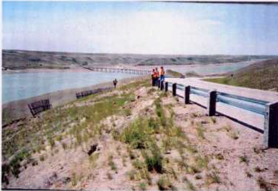
Photo 1 – View of downslope edge of the road above slide area (2001). Note newly-installed guardrail and slide scarp visible downslope of road.
