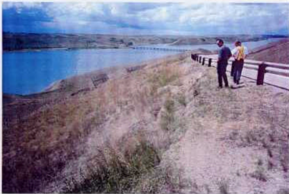
Photo 2 – Downslope edge of road as seen during the June 2000 assessment.
