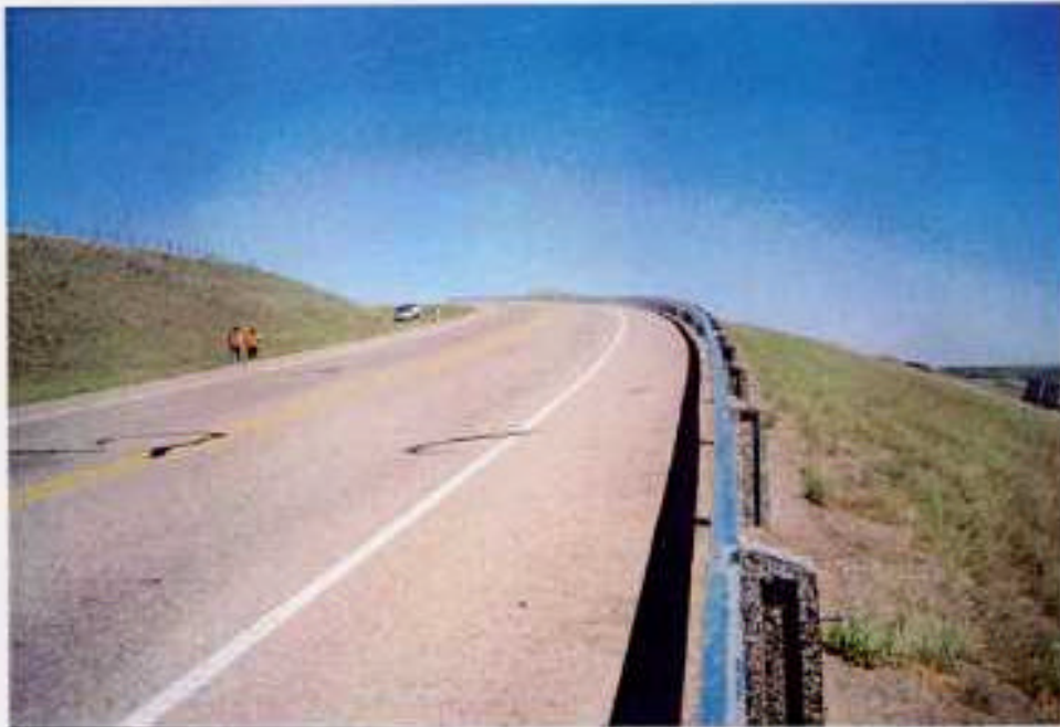
Photo 3 – Facing northeast along road through slide area. Note newly-installed guardrail.
