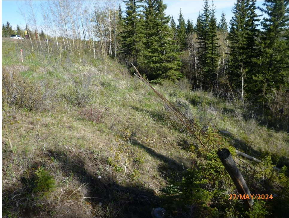
Photo 5 Downslope of the pile wall. Fence knocked over from slope movement. Photo taken facing north on May 27, 2024.
