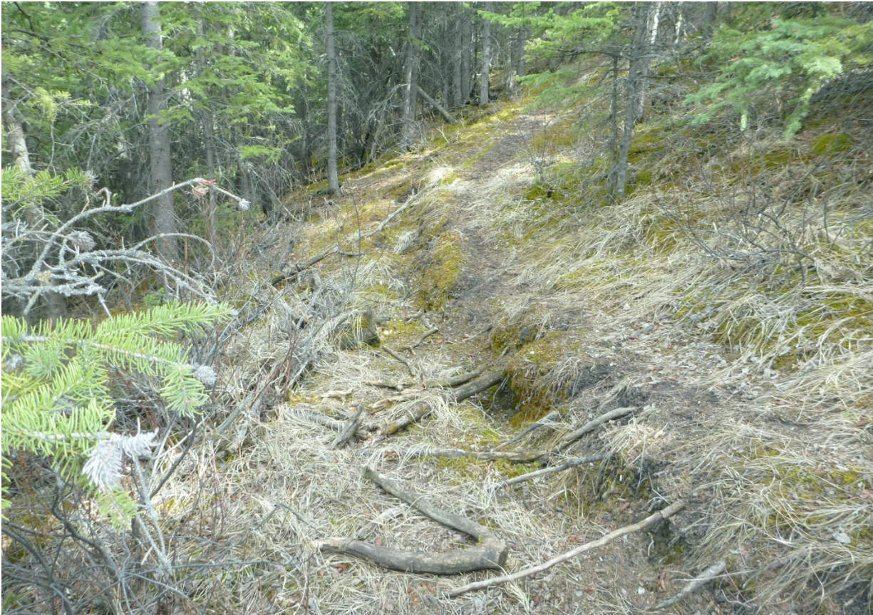
Photo 5 Slope movement in forested area to the east of the highway. Photo taken facing south on May 7, 2019.
