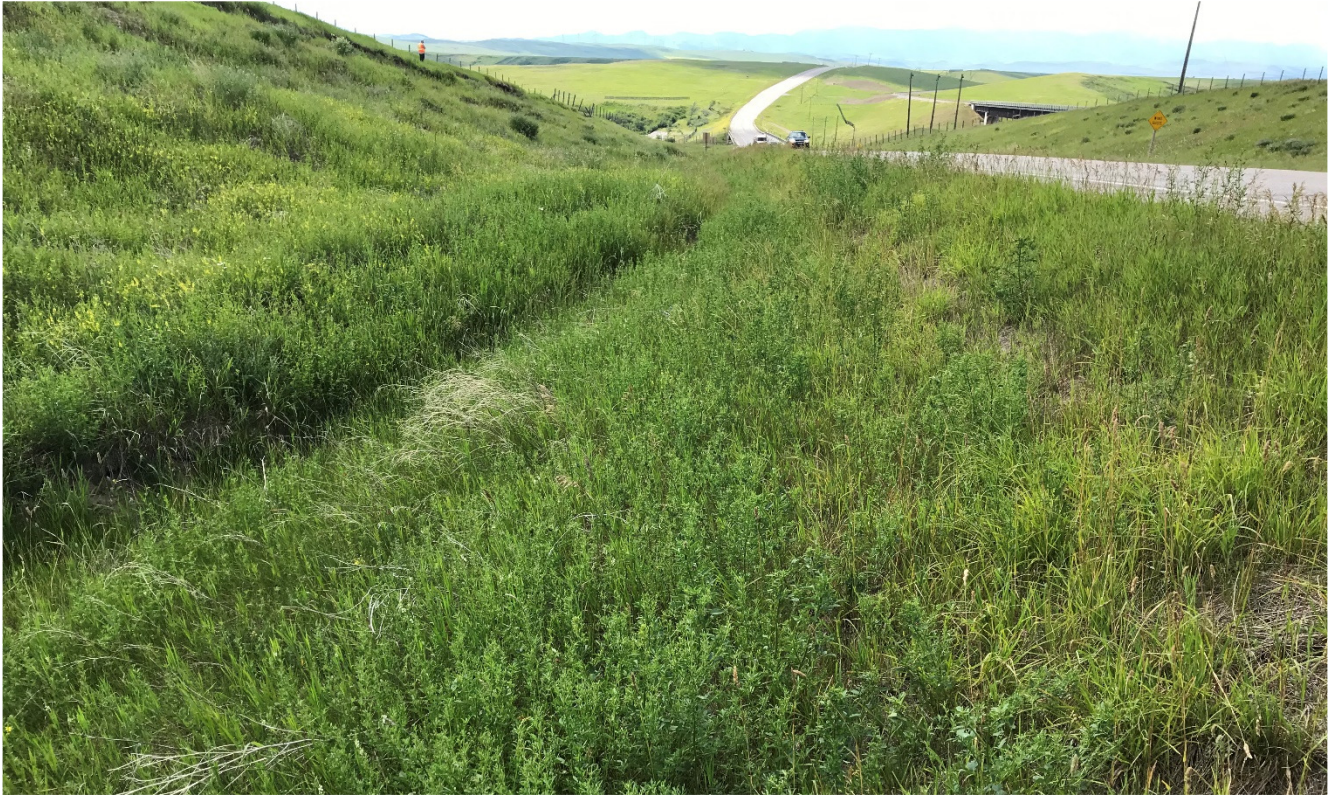
Photo 3 Toe rolls blocking the ditch. Photo was taken facing west on July 8, 2021.
