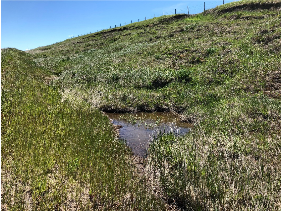
Photo 5 Toe rolls blocking ditch at several locations. Photo taken facing east on June 9, 2020.
