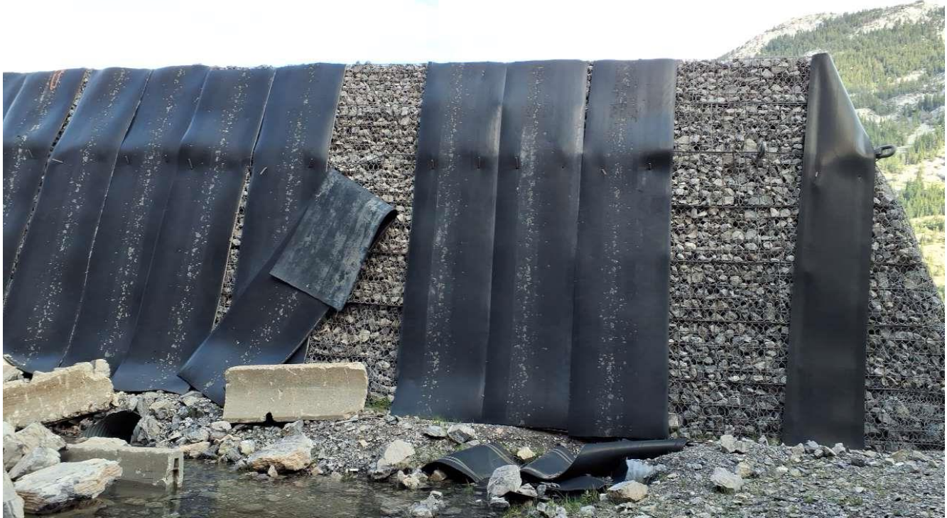
Photo 7 Rubber mats on south side of gabion wall have become detached and should be reinstalled to protect gabions from rockfall damage. Photo taken facing north on May 30, 2024.
