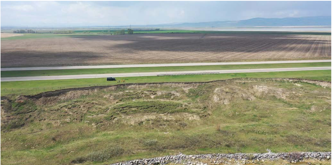
Photo 1 Slide area. Photo taken facing west on May 10, 2023.
