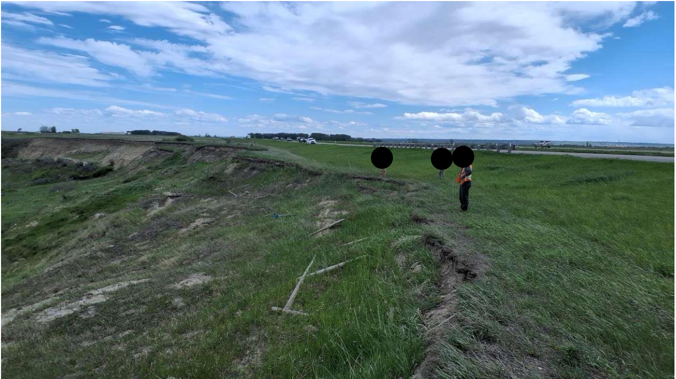
Photo 3 Head scarp located up to 5 m past the fence line. Photo taken facing south on May 29, 2024.
