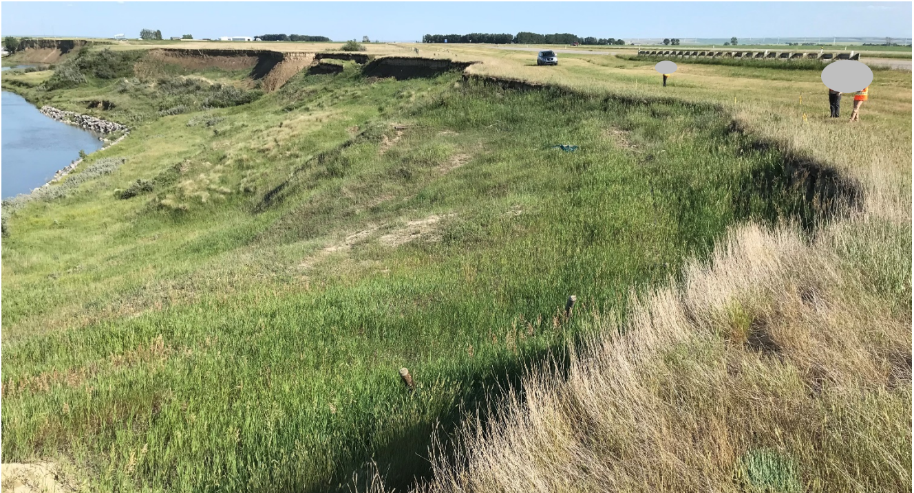
Photo 3 Ongoing slide movement retrogressing towards the highway. Photo taken facing southeast on July 8, 2021.
