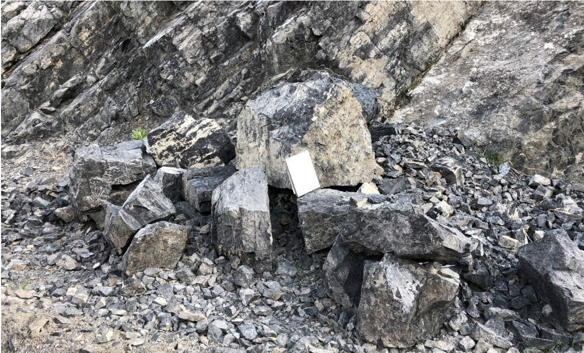
Photo 5 Rockfall debris up to 3.5 m 3 in the ditch of Site B. Photo taken May 17, 2022, facing northwest.
