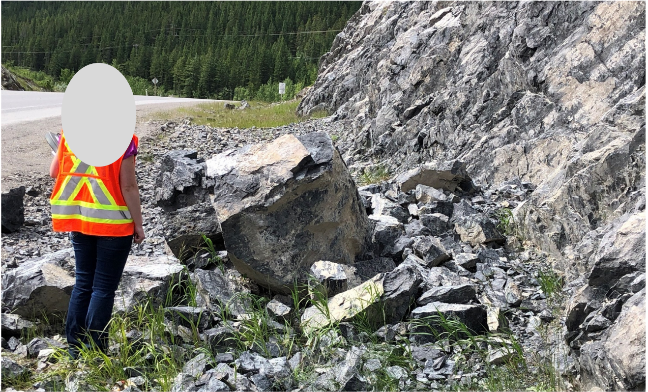
Photo 5 Rockfall debris up to 0.25 m 3 in the ditch of Site B. Photo was taken facing northwest on July 6, 2020.
