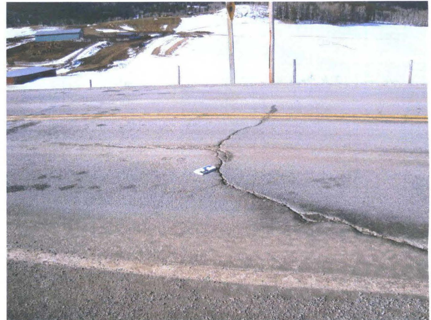
Photograph 5 – Looking west at the arc shaped cracks in the road surface.
