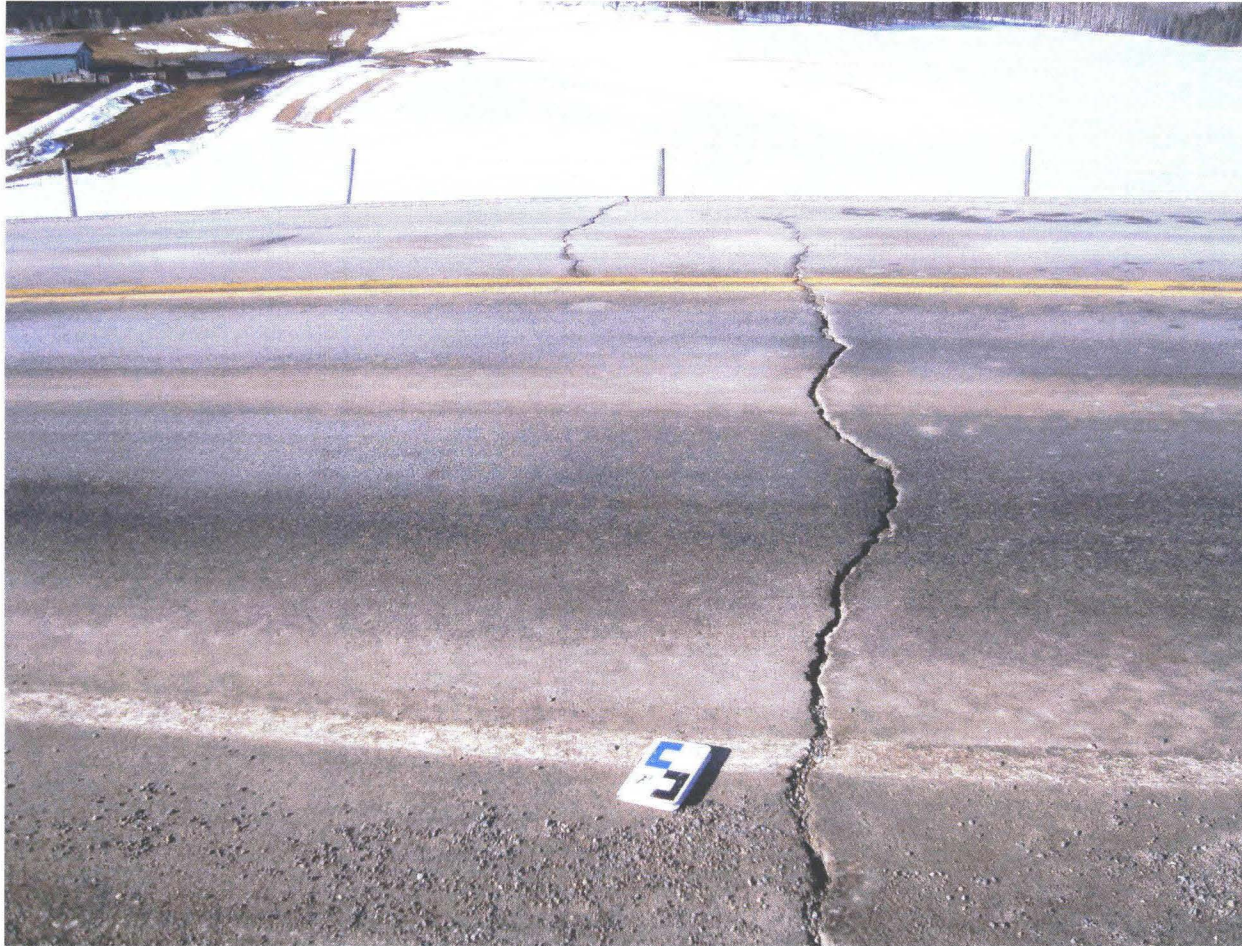
Photograph 6 – Looking west at the cracks perpendicular to the direction of travel.
