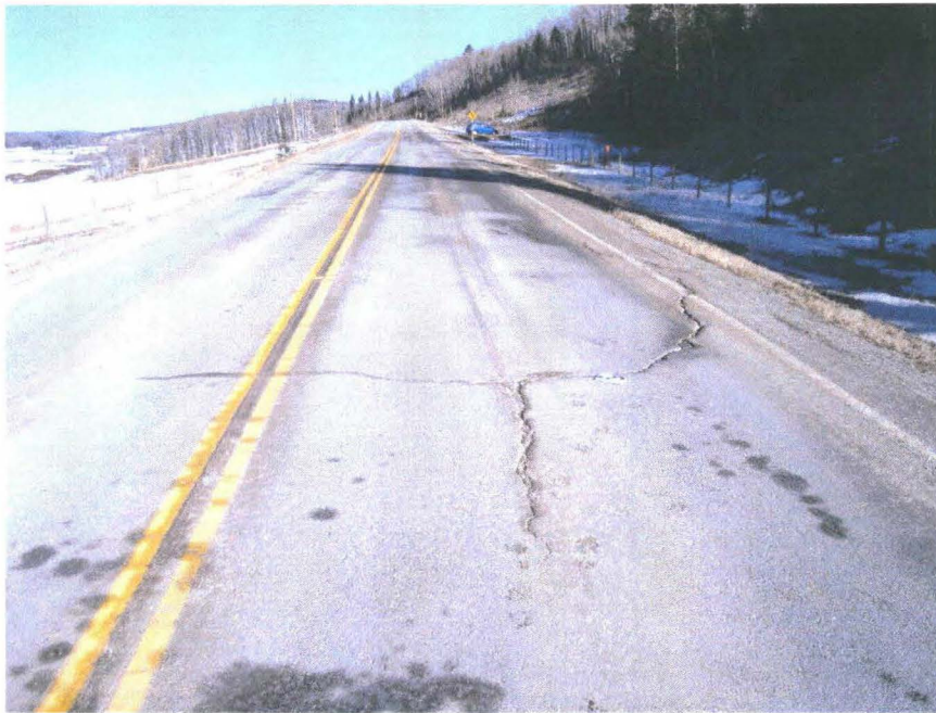
Photograph 4 - Looking north towards the arc shaped cracks in the road surface. Field notebook shown for scale.
