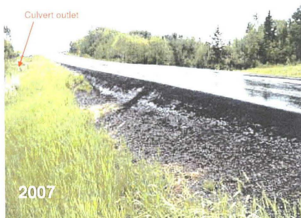
Photo S10(C)-3 – June 2007 (lower left) Closer view of the edge of the recent overlay, along the east shoulder of the road. The approximate location of the culvert to the south of the overlay is shown.
