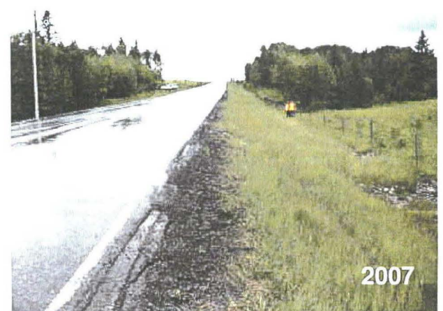
Photo S10(C)-4 – June 2007 (lower right) Facing south along the west shoulder of the road. The culvert shown in Photos S10(C)-5 and 6 is just behind the two people standing in the ditch to the right of the road.
