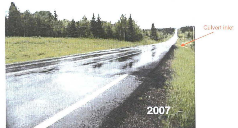
Photo S10(C)-2 – June 2007 (upper right) Typical view facing north across the recent overlay at the site, as seen during the June 2007 site inspection. The approximate location of the culvert to the south of the overlay is shown.
