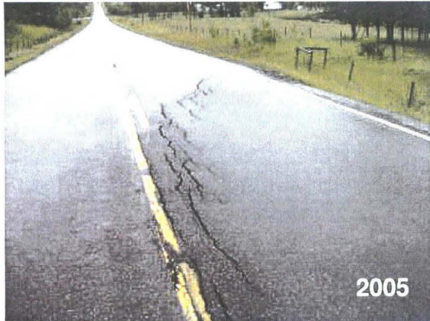
Photo S10(C)-1 – June 2005 (upper left) Cracking and settlement of the road surface as observed during the 2005 site inspection.
