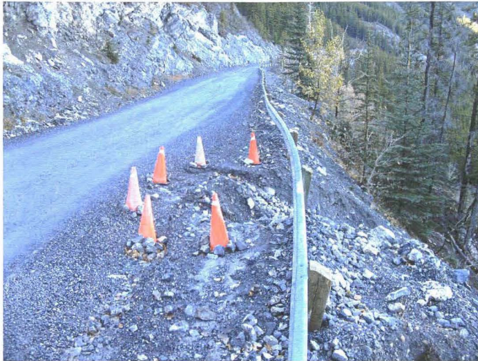
Photo 742-32 (top) – At ~Km 5.7, gully erosion in the fill slope below the road that has encroached below the guardrail and reduced the trafficable width of the road. Debris from plowing and grading the road surface has built up below the guardrail in the segment of the highway upslope /southbound from this location and has caused a concentration of surface runoff to discharge onto the fill slope below the road at this location, which has led to the gully erosion.
