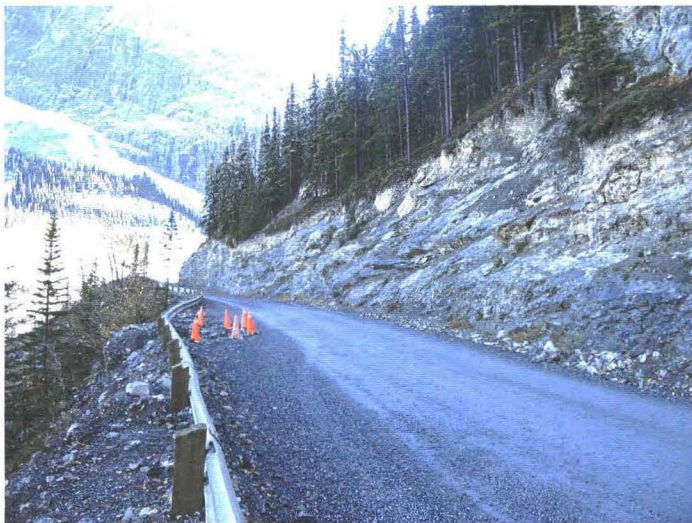
Photo 742-33 (middle) – Facing southbound towards the gully erosion and illustrating the reduction in road width adjacent to the gully.
