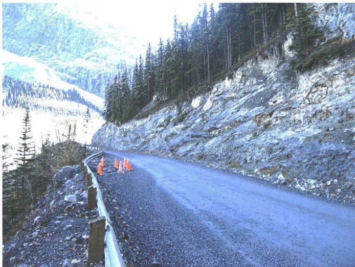
Photo 742-33 (middle) – Facing southbound towards the gully erosion and illustrating the reduction in road width adjacent to the gully.
