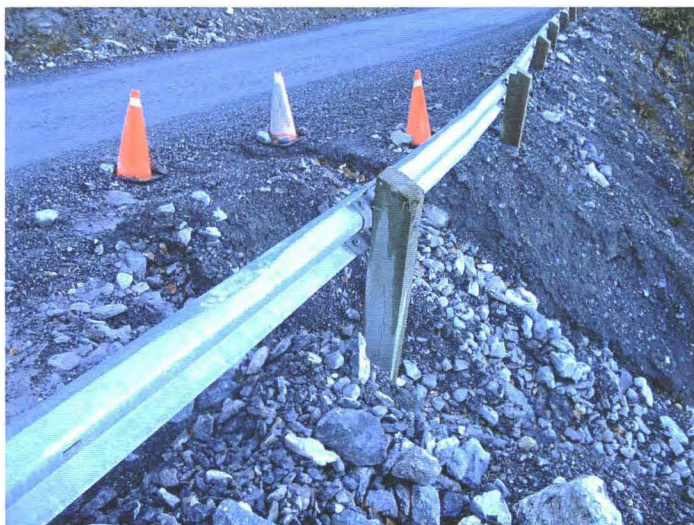
Photo 742-34 (bottom) – Another view of the head of the gully erosion, showing how the guardrail posts have been undermined.
