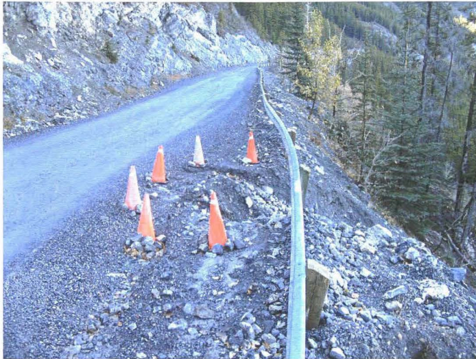
Photo 742-32 (top) – At ~Km 5.7, gully erosion in the fill slope below the road that has encroached below the guardrail and reduced the trafficable width of the road. Debris from plowing and grading the road surface has built up below the guardrail in the segment of the highway upslope /southbound from this location and has caused a concentration of surface runoff to discharge onto the fill slope below the road at this location, which has led to the gully erosion.
