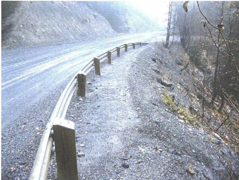
Photo 742-16 (top) – Opposite the drainage draw at Km 4.1, showing the guardrail inset more than 1 m from the crest of the fill slope below the road.
