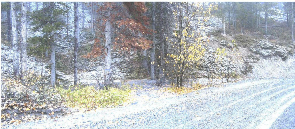
Photo 742-17 (bottom) – Drainage draw upslope of the road at approximately Km 4.15, infilled with sediment and water from the ditch flow similar to the draw at ~Km 4.1.
