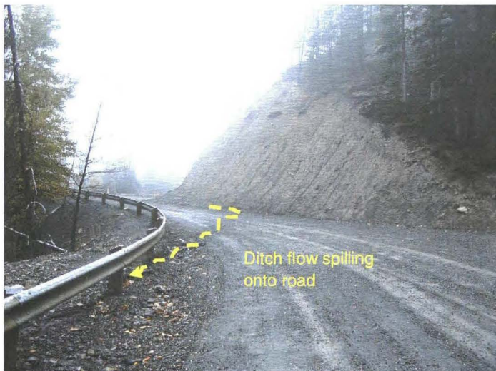
Photo 742-13 (bottom) – Facing southbound from approximately Km 4.2, with the ditch flow coming across the road surface as shown. A typical cut slope in the order of 8 to 9 m high and up to 45° inclination is visible in the background.
