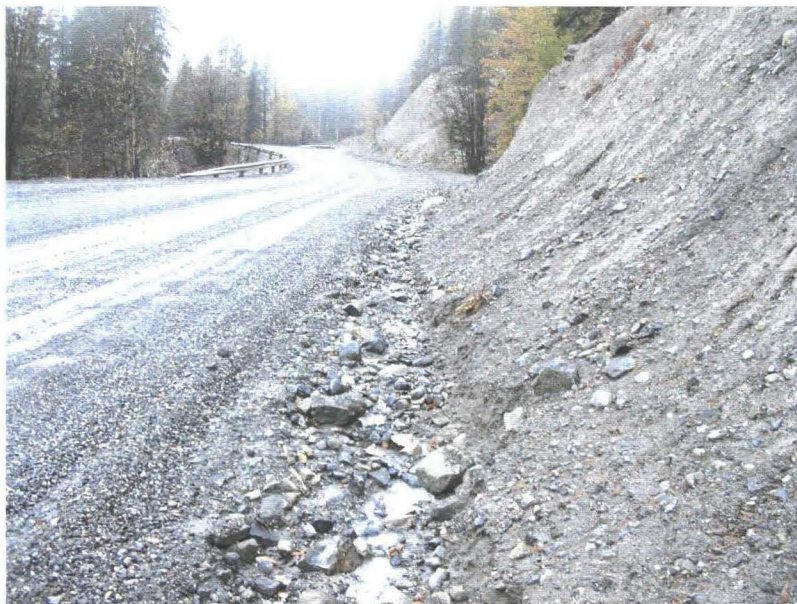
Photo 742-10 (bottom) – Facing southbound/uphill along the ditch immediately northbound of the Km 4.1 Drainage Draw. The slope wash/eroded material along the toe of the cut slope has filled the very small ditch. The ditch flow has washed the fine grained soil from the material and left behind the gravel-sized and larger rocks behind.
