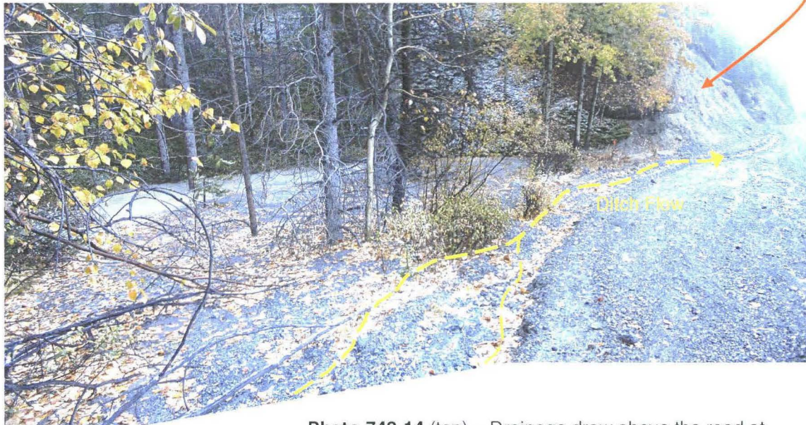
Photo 742-14 (top) – Drainage draw above the road at ~Km 4.1, infilled with sediment and water from the ditch flow. There does not appear to be a culvert installed at this location. The ditch flow appears to continue past this location, as marked. Note the dead tree in the infilled area.
