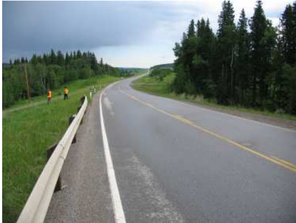
Photo S7-5 – June 2007 (upper left) Facing east across the segment of the highway where the shear keys were installed in 2004 (approximately Sta. 5+400/5+460) in order to prevent further landslide damage to the highway. Aside from one crack in the road surface (shown in Photo S7-6), there has been no further damage to the road surface since the repair.
