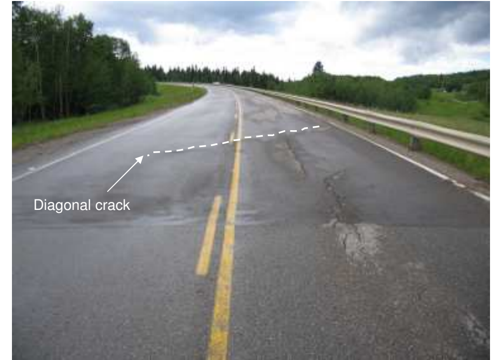
Photo S7-6 – June 2007 (upper right) Facing west across the segment of the highway where the shear keys were installed in 2004. The diagonal crack visible in the middle background (highlighted in the photo) has developed since the repair, but otherwise no further damage to the road surface. There was negligible vertical displacement across the crack at the time of the inspection.
