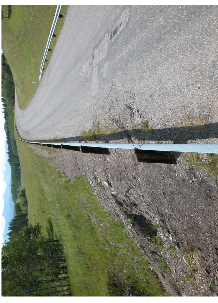
Photo S13-2 (upper right) – July 2003 – same area as shown in Photo S13-1, as seen during the July 2003 inspection.
