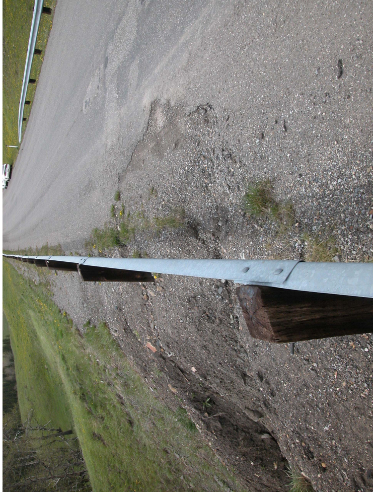
Photo S13-1 (upper left) – May 2004 – gully erosion retreating into the south edge of the road surface. There has been a slight retrogression (estimated less than 5 cm) of the erosion further back into the road since the July 2003 inspection. Compare with Photo S13-2.
