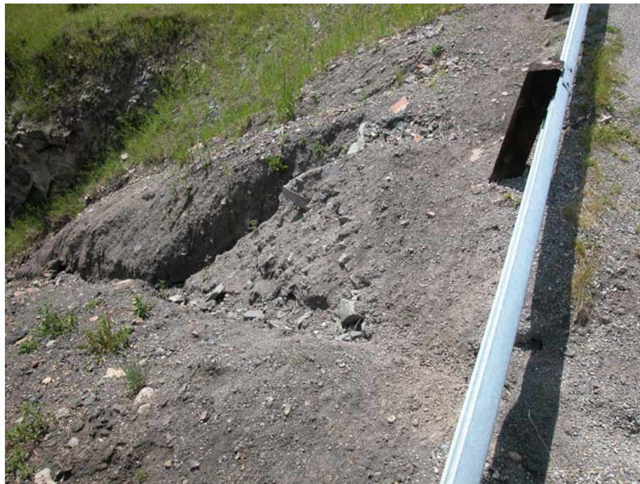
Photo 4 (upper left) Another view of the gully erosion immediately south of the guardrail, showing the proximity of the steep drop-off to the road.
