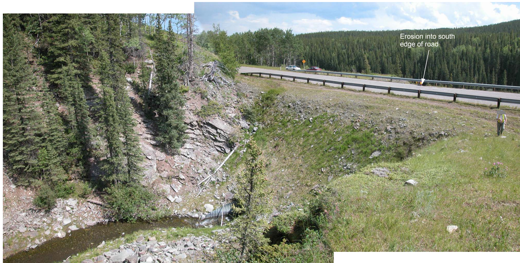
Photo 7 (top) General view of the creek to the north of the highway. The culvert inlet is visible in the center, bottom of the photo. The point on the south guardrail shown in Photos 3 and 4 is as shown.
