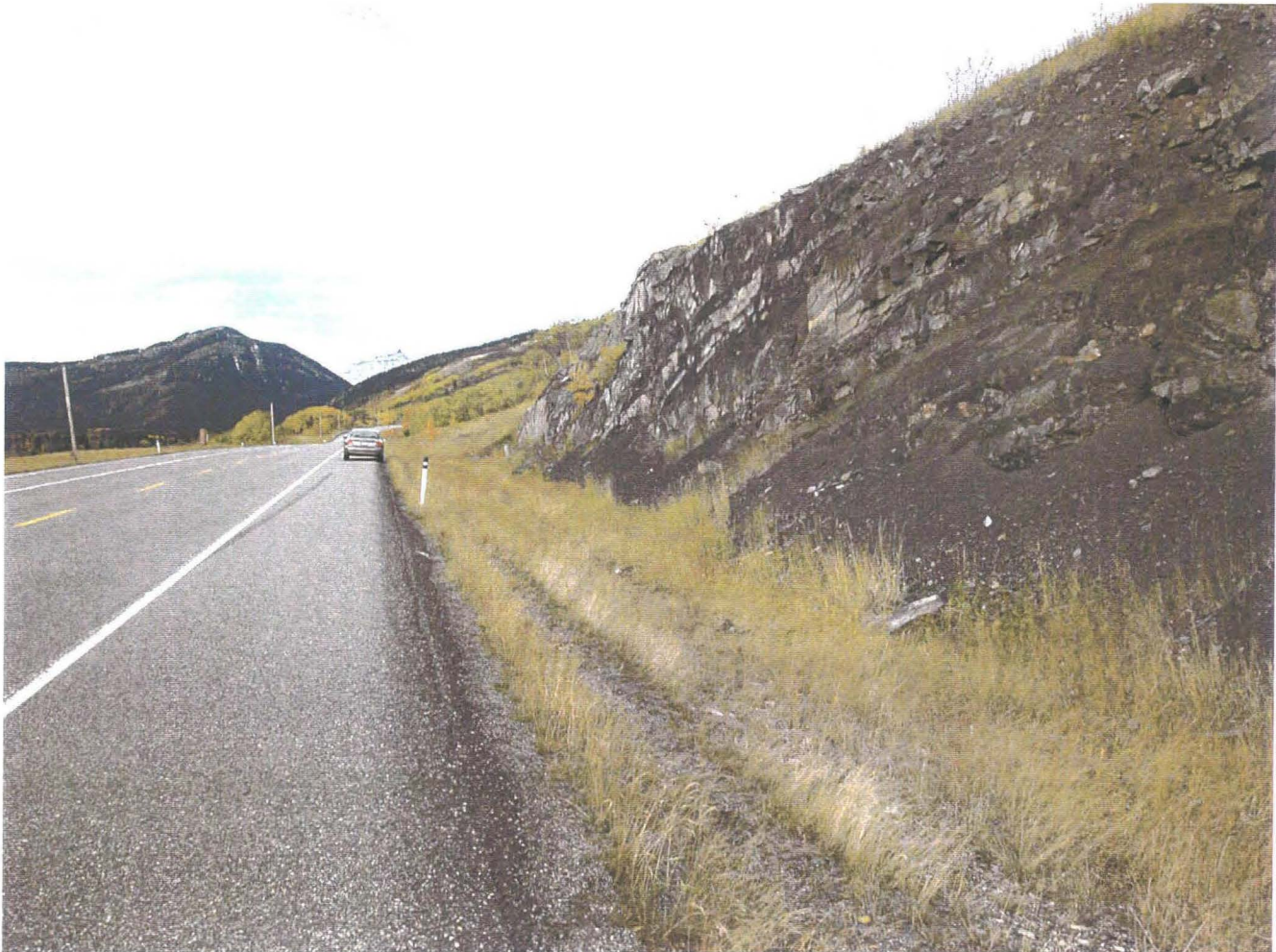
Photo 1 – Facing west along Highway 541 at the Highwood River Recreation Area Rock Cut site. Rockfall debris from the cut slope has accumulated along the toe of the slope. There were no signs of rockfall damage to the road surface and the existing ditch appears to be of sufficient size to contain the rockfall debris provided that it is cleaned out as necessary.
