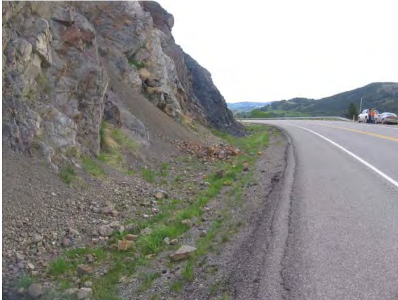
Photo 3 (top) – June 2009 Facing eastbound along the north ditch, showing the accumulation of rockfall debris along the ditch.
