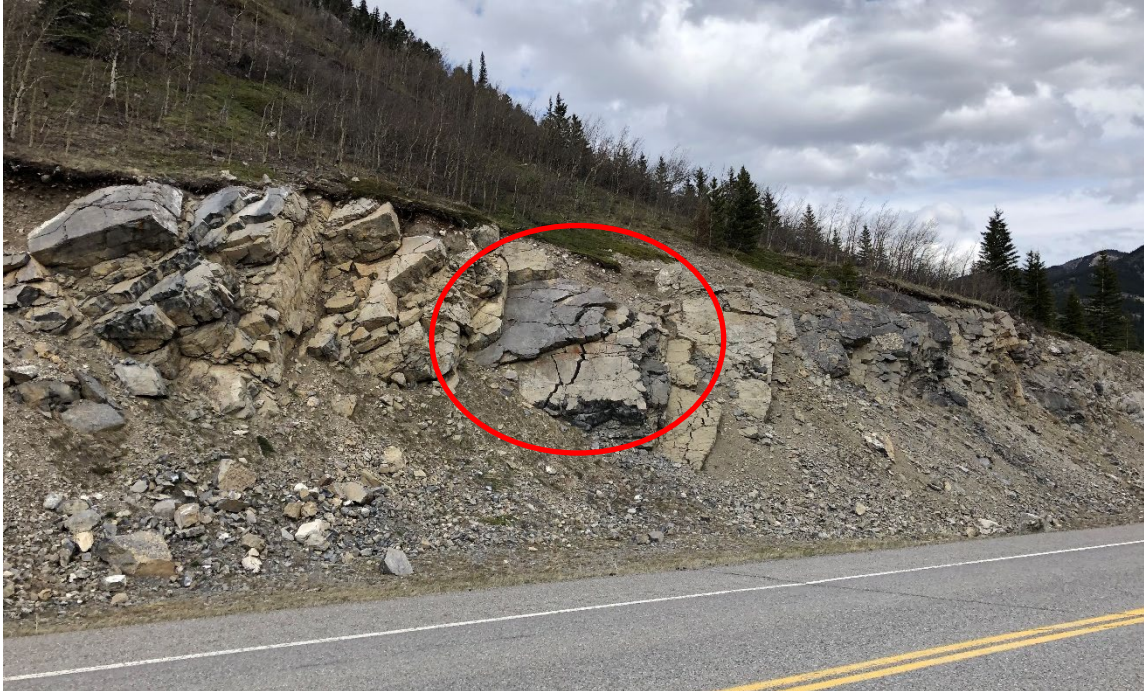
Photo 7 Bedrock fracturing at S070-III (indicated by red circle) leading to future rockfall blocks. Photo taken May 16, 2022, facing northeast.
