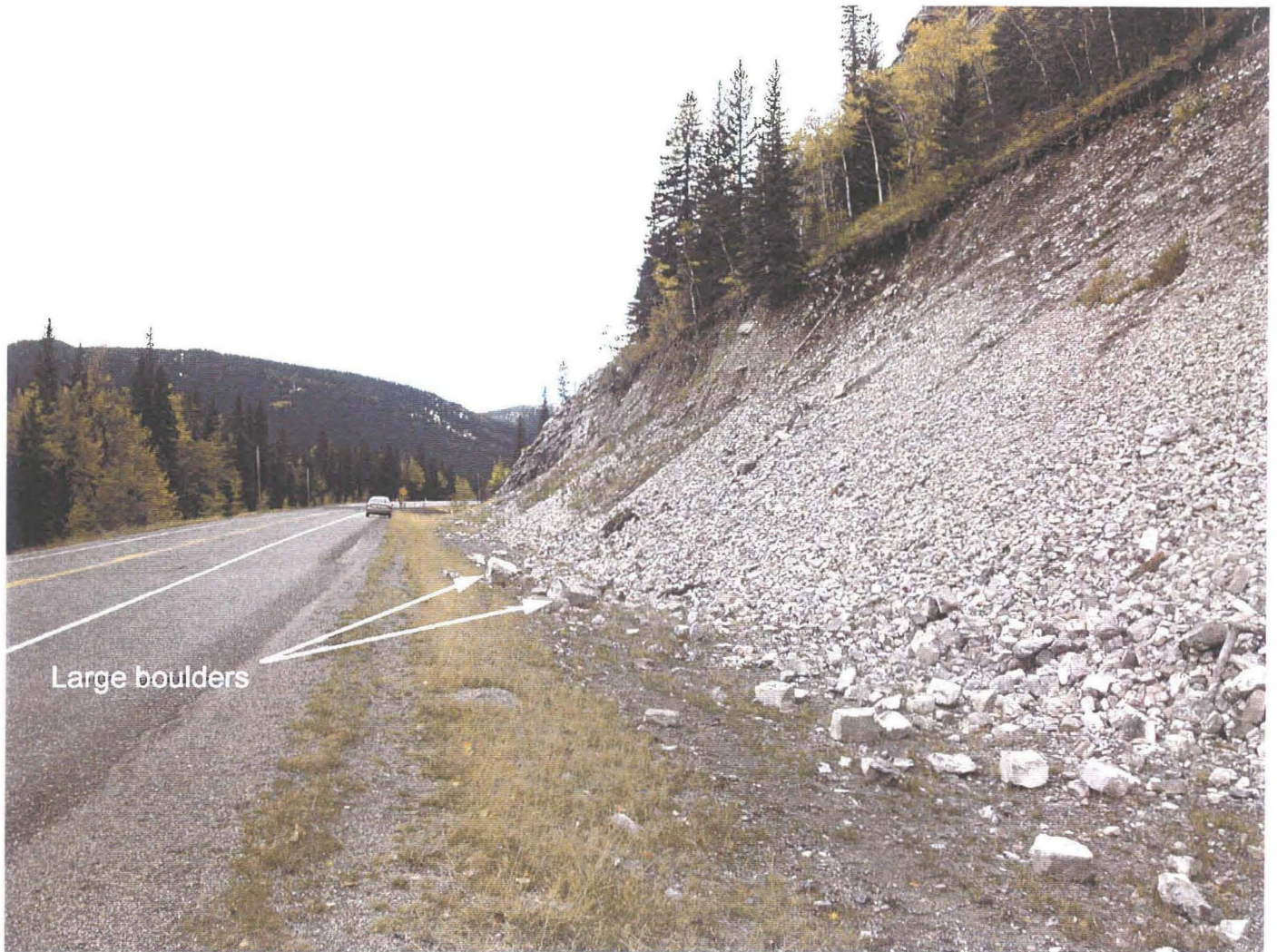
Photo 1 – Facing west along the ditch at the toe of the colluvium slope. Cobble to boulder sized rocks have rolled beyond the toe of the slope, however there were no rocks on the road or signs of rockfall damage to the pavement. Two large boulders (approximately 1.5 m maximum dimension) were noted within 3 m of the edge of the pavement. There were no other boulders of comparable size visible in the debris and it is not entirely clear if these boulders actually originated from the cut slope.
