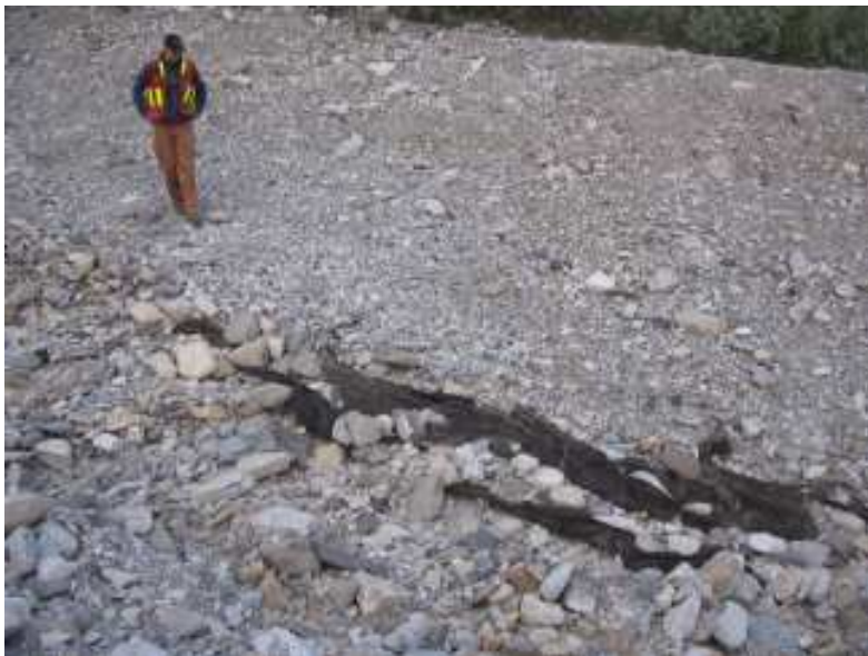
Photo S21-5 (bottom) – June 2008 Geotextile exposed along the channel upstream of the culvert inlet.
