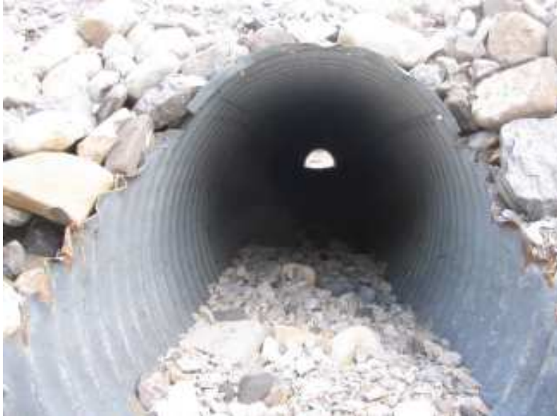
Photo S21-4 (top) – June 2008 Facing upstream from the culvert outlet, with debris accumulation in the pipe.
