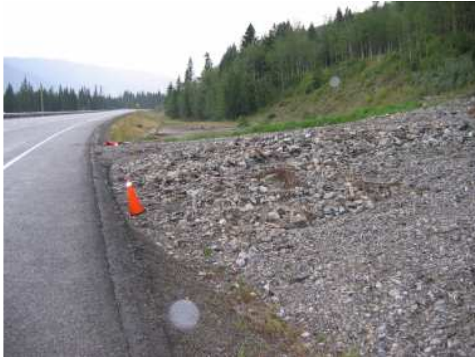
Photo S21-1 – August 2004 (upper left) Facing west across debris filling the north ditch and burying the culvert inlet. It appears that the debris had previously buried the culvert inlet and also extended onto the westbound lane of the highway before being cleared by the maintenance contractor.
