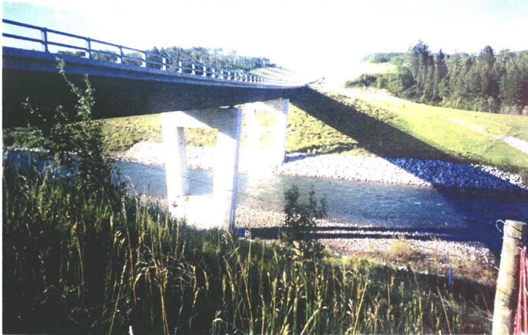
Photo 3 – Looking south at south abutment. Note erosion protection works in west ditch of the abutment fill.
