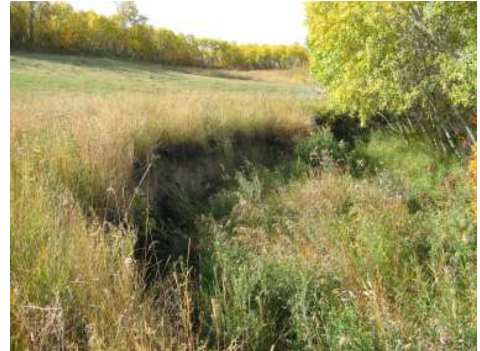
Photo S23-5 – September 2006 (right) Landslide scarp in the vicinity of SI #5 around the upper east flank of the landslide area (see Figure S23-2 for an illustration of this location). This 2 to 2.5 m high, near-vertical scarp has presumably formed since SI #5 was installed in 1990 because the SI is located at the base of the scarp at a location that would not be accessible for the drilling equipment with the scarp in place.
