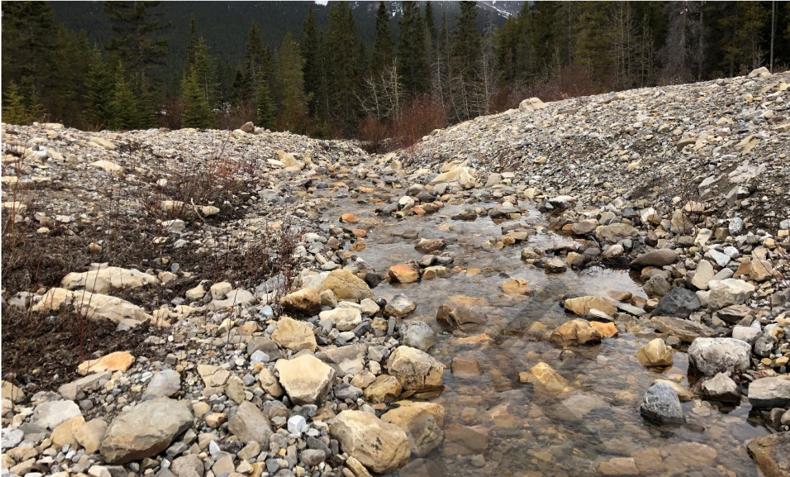
Photo 3 Culvert discharge on west highway embankment slope. Photo taken May 17, 2022, facing west.
