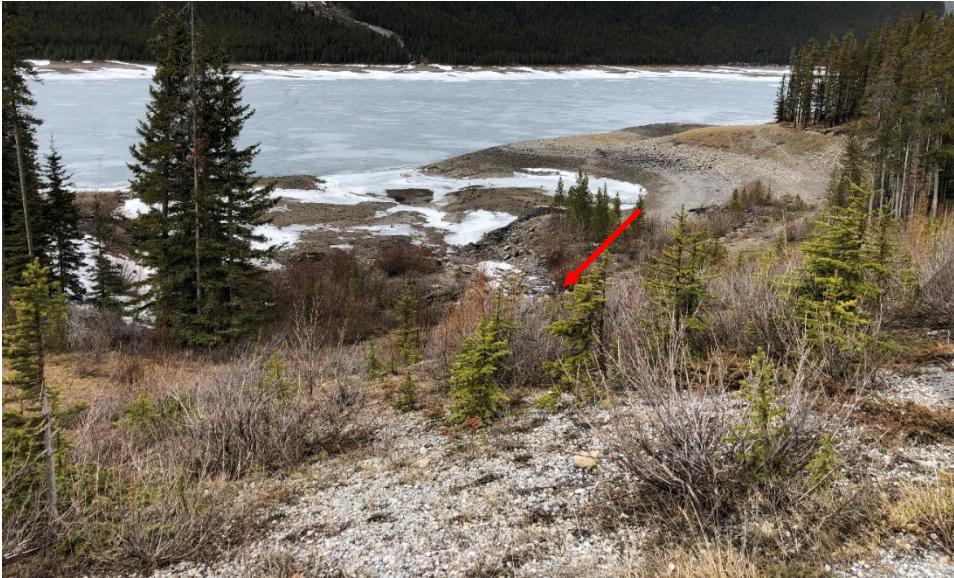
Photo 6 West highway embankment slope. The outlet of the 2 m diameter CSP culvert is indicated by red arrow. Photo taken May 17, 2022, facing northwest.
