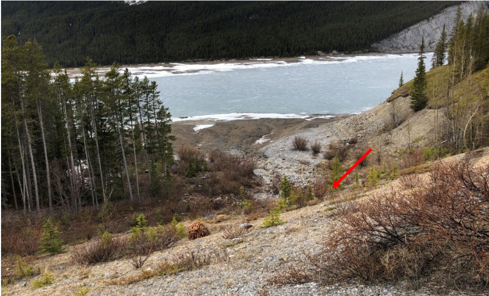
Photo 3 West highway embankment slope. The outlet of the 2 m diameter CSP culvert is indicated by red arrow. Photo taken May 17, 2022, facing northwest.
