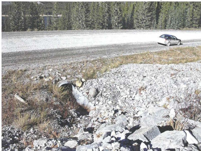
Photo 742-48 (top) – Facing downslope along the creek channel towards the culvert inlet. Note the debris extending northbound (to the right) along the ditch.
