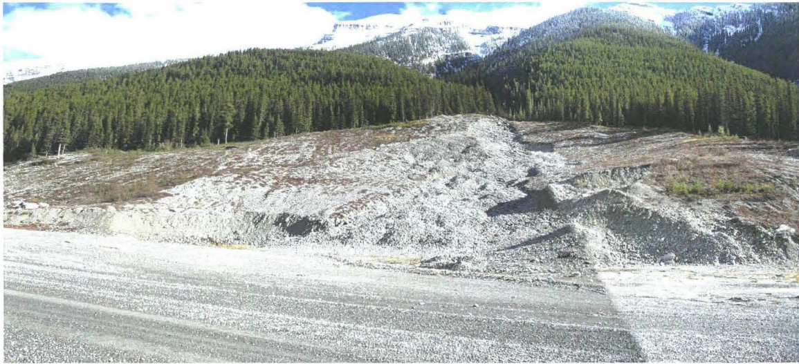
Photo 742-38 (top) – Facing northeast along the seasonal creek channel. The surface channel tapers out a short distance upslope of the highway and it appears that any seasonal flow along the creek percolates down into the fan and flows below the highway.
