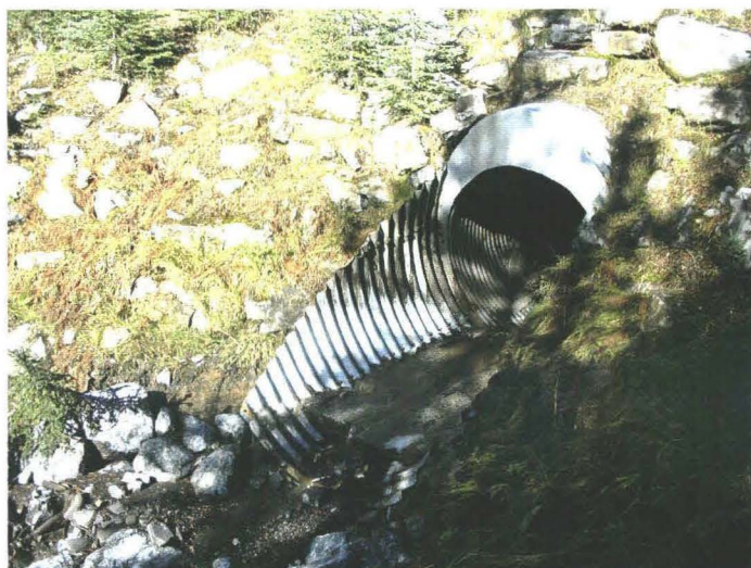
Photo 742-59 (bottom) – Culvert outlet below the highway. Note the debris accumulation along the base of the culvert.
