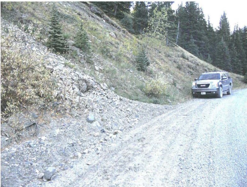
Photo 940-50 (top) – Facing northbound across the toe of the cut slope. Note how the debris from the gully extends to the upslope edge of the road and overflows from the negligible ditch. The lowermost portion of the fan had been graded out to clear the road earlier in 2008.
