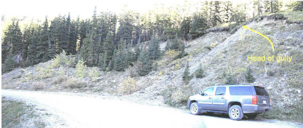
Photo 940-48 (top) – General view of the cut slope along the highway. Note that the gully headwall is around the crest of the cut slope, i.e. the gully runs the entire length of the cut slope.
