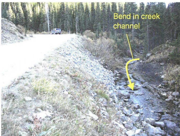
Photo 940-46 (middle) – Closer view of the 2008 repair area, facing southbound along the highway and upstream along the creek. Note how the repair area is a short distance downstream of a bend in the creek channel.
