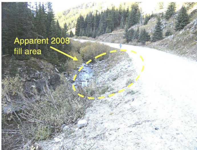
Photo 940-45 (top) – Facing northbound along the highway and downstream along the creek. The rock fill area that appears to have been placed in 2008 to buttress the downslope edge of the road is marked.
