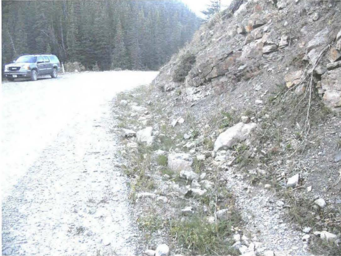
Photo 940-44 (bottom) – Facing northbound along the toe of the cut slope. Note the very small ditch, and the cobble-sized rocks that have fallen from the cut slope.
