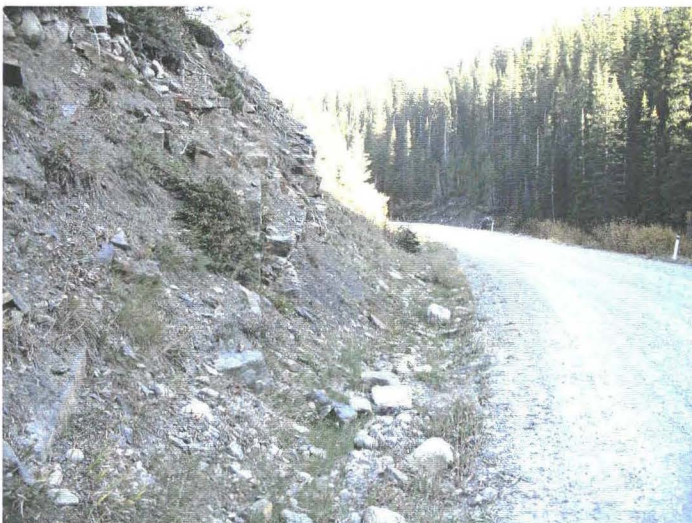
Photo 940-43 (middle) – Facing southbound along the toe of the cut slope. Note the very small ditch, and the cobble-sized rocks that have fallen from the cut slope.
